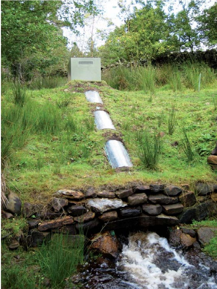
A buried 1 kW screw at Bonfield Ghyll, North York Moors National Park (photo: MannPower)
