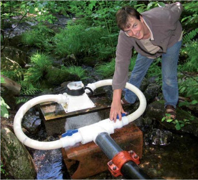
A DIY 'pico' hydro power installation in Canada
