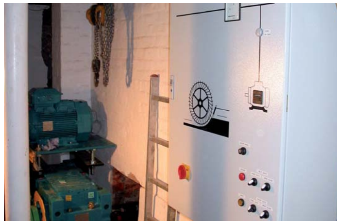
Electrical control panel at Lemsford Mill, Hertfordshire (photo courtesy Ramblers Worldwide Holidays)
