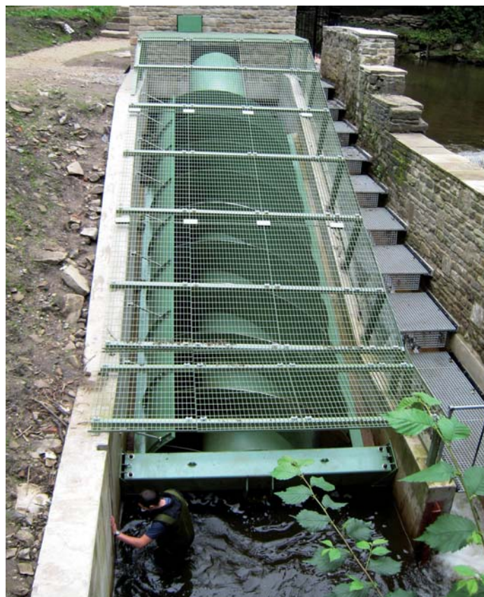
An Archimedes screw at the Torrs hydro scheme at New Mills in High Peak provides cheap and plentiful power to local business and homes (photo: MannPower)
